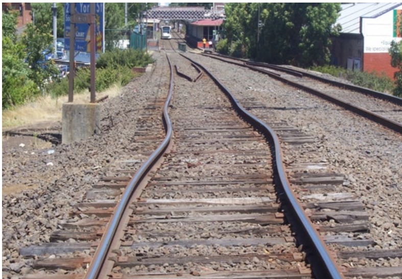
FIGURE 3: Rail buckling due to high ambient temperatures
